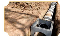
Sewage Treatment Plant
